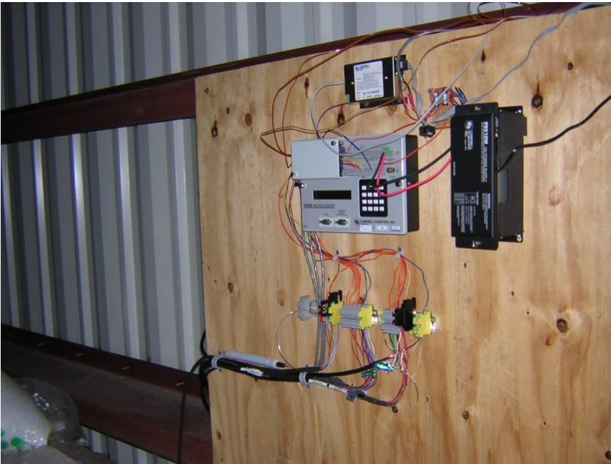
Figure 5-Roof Sensor Wiring and Datalogger
